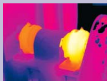
Overheating bearing cap
